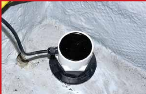
Photo 23: once set (24 hours +), the transducer assembly is screwed into position with a good big dollop of Fix-A-Tap lubricant on the face. But before doing so, wind it anti-clockwise a number of turns so that the cable ends up without loops or kinks. Screw down as hard as you can with your fingers, but don't force it. Lace any loose cables.
